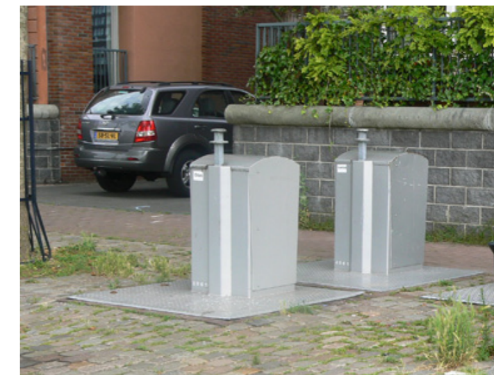
Example of service boxes/metering cupboards which are visible and easily accessible, yet in keeping with the colour palette used in this development
