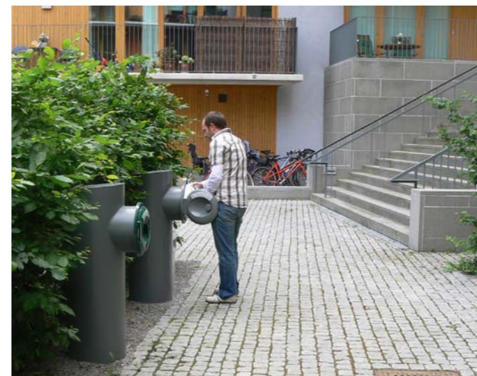
The Envac refuse system in Hammarby and Malmo, Sweden, segregates commercial and domestic waste, which are transported underground by vacuum suction to central collection points
